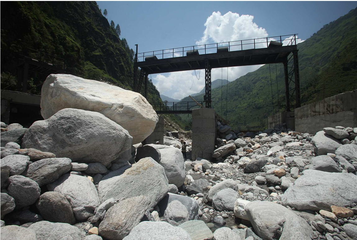
Figure 7: Boulder bed-load upstream of the destroyed 5 MW Himalaya Hydro Tanga HEP on Paina gad.
